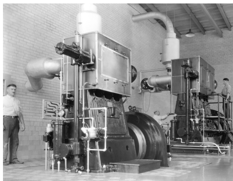
Interior of the new powerhouse
